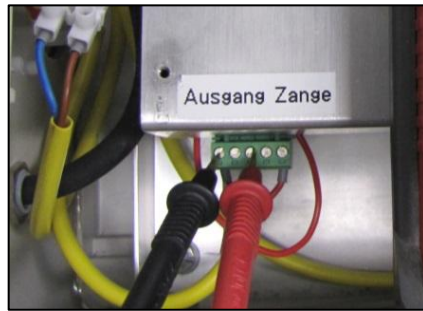
Fig. 9-3 Head stunning voltage measurement E6 and E8
