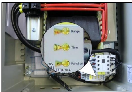
Fig. 5-4 Timer relay in transformer TR7
